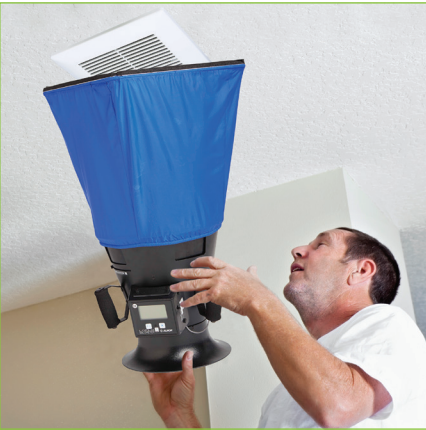
Balometer used to verify installed performance
